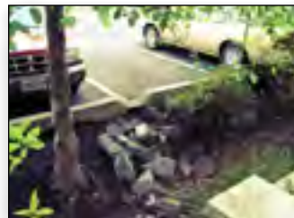
Water runoff from surface parking can be handled in various ways including edge treatment, islands, etc.
