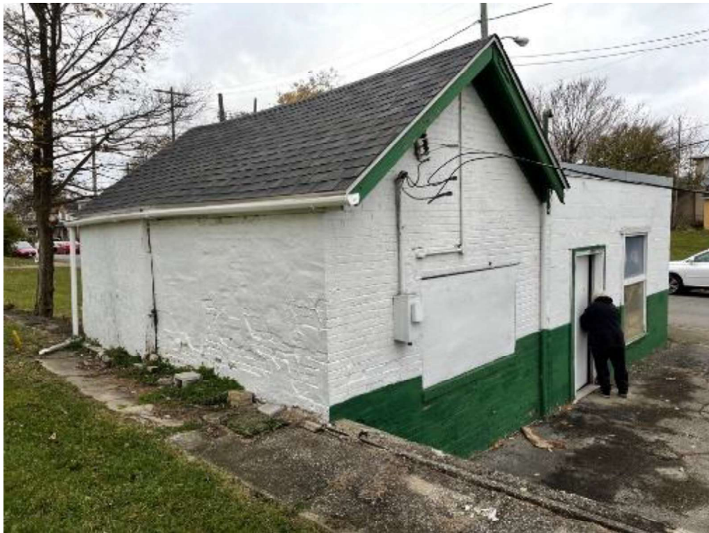
View Facing Southeast Elevation – Original Brick Building with Gabled Roof in Foreground
