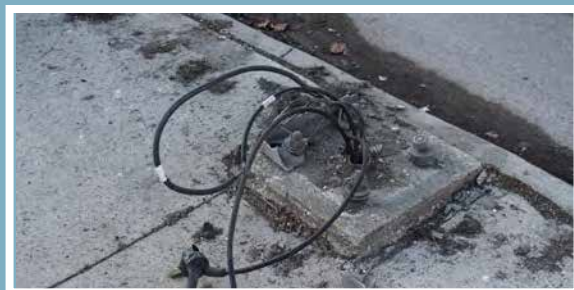
LACK OF PEDESTRIAN-SCALE LIGHTING
