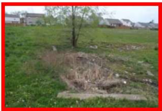
Figure 8a: The view to the west from the 18" inflow pipe at the southeast corner of the basin
