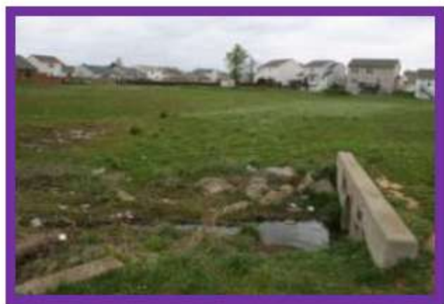
Figure 8c: The view to the north from the 18" inflow pipe at the southeast corner of the basin
