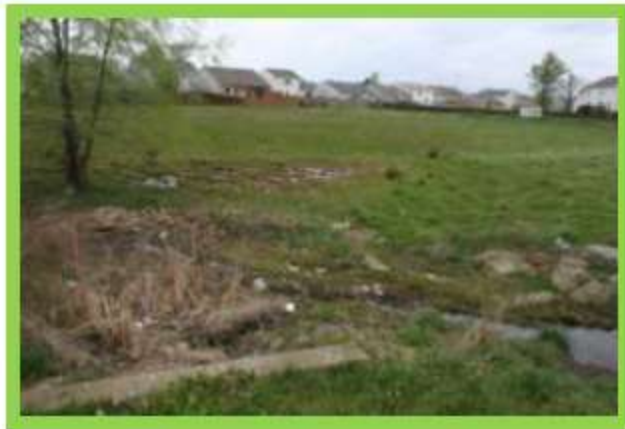
Figure 8b: The view to the northwest from the 18" inflow pipe at the southeast corner of the basin
