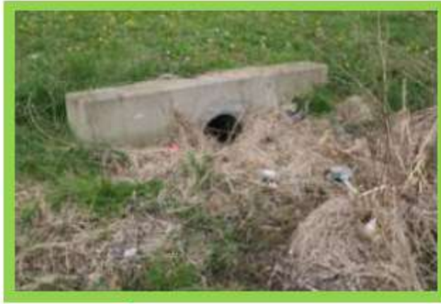
Figure 9b: 18" inflow pipe
