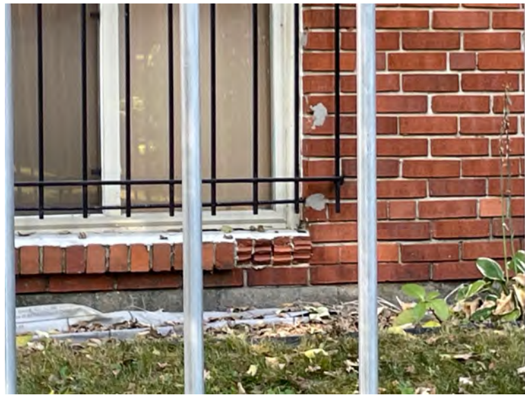
Broken window pane
