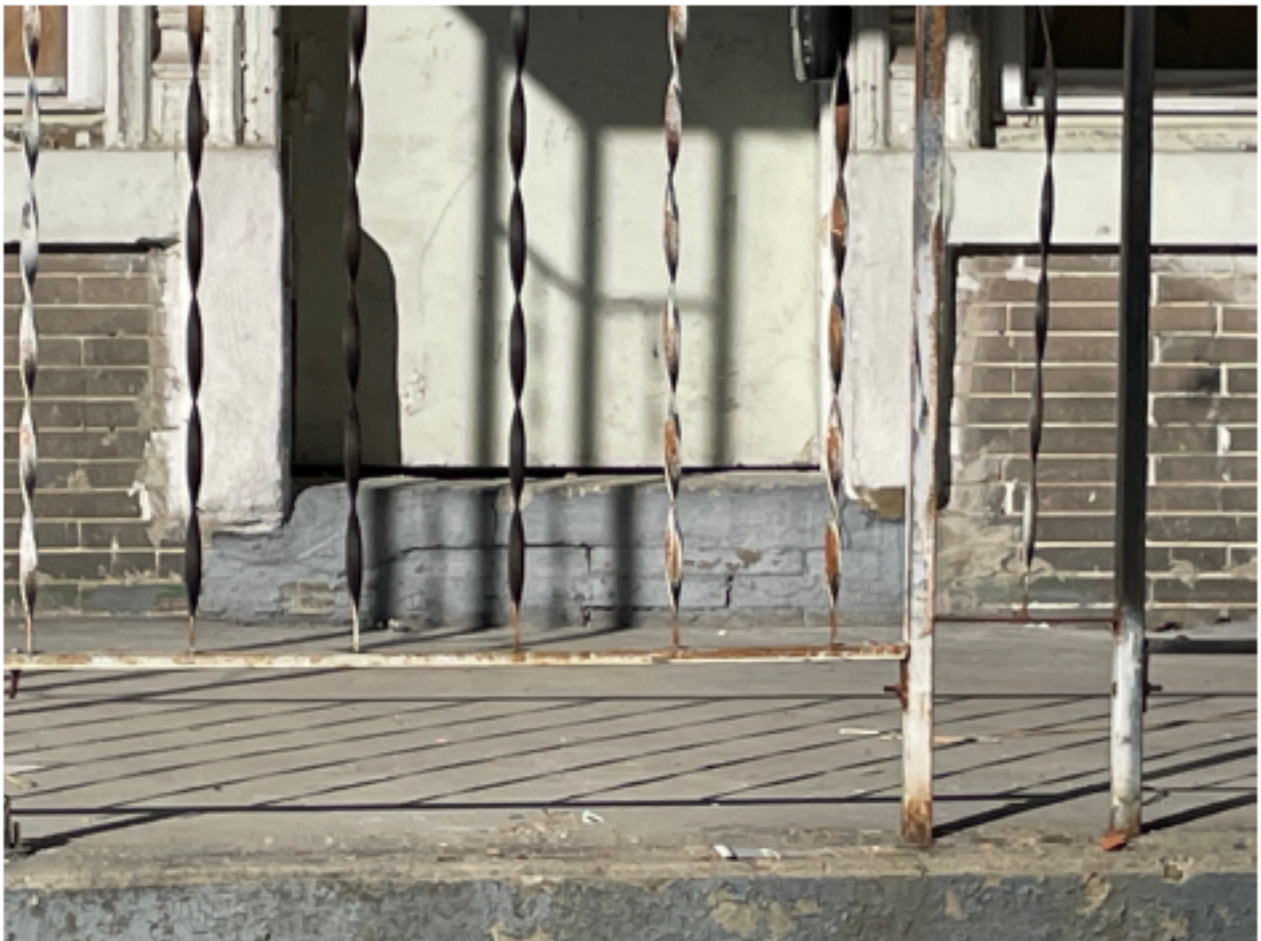
Missing threshold components with gapping under front entry door
