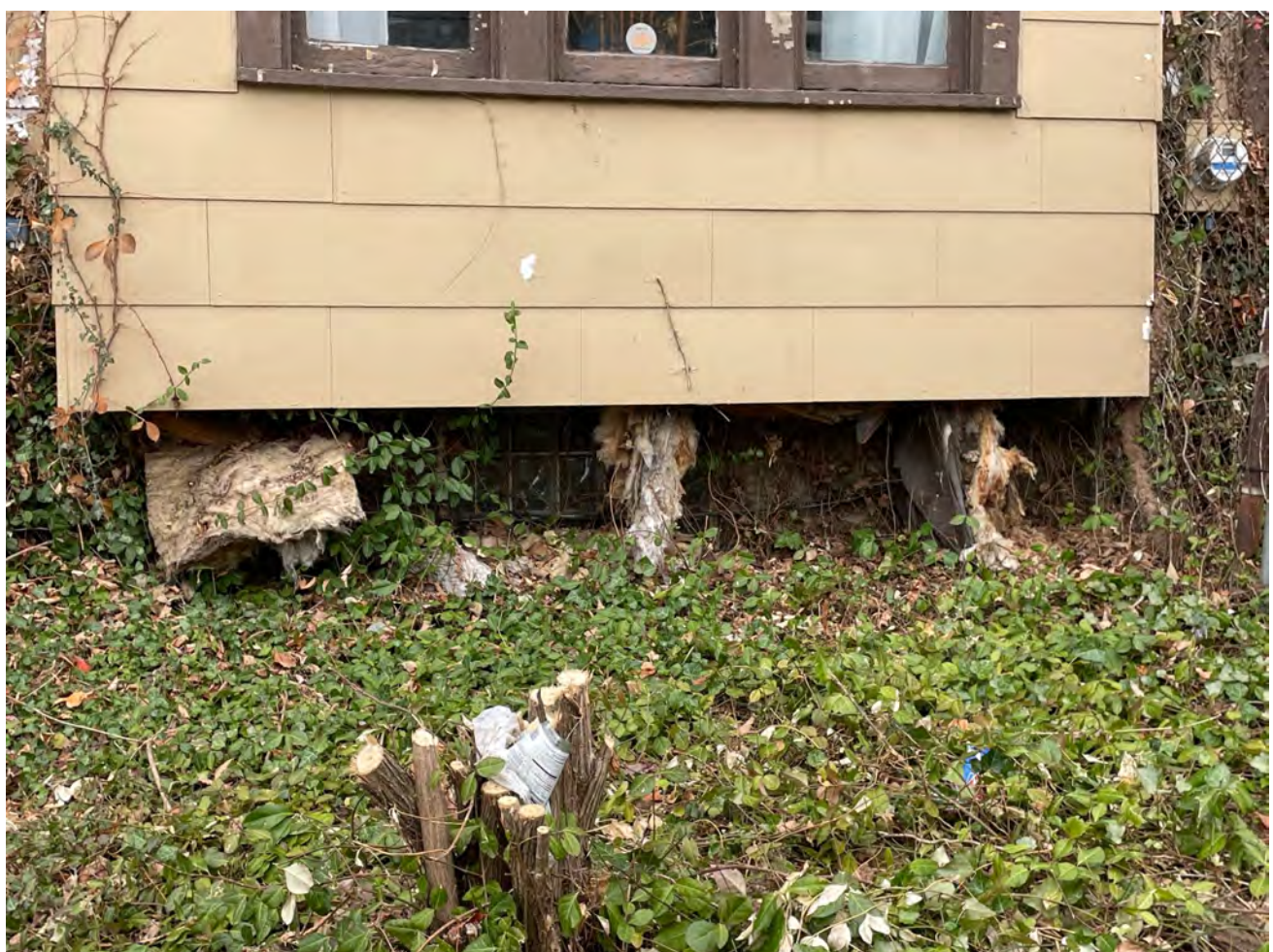
Detached insulation materials under south side of structure
