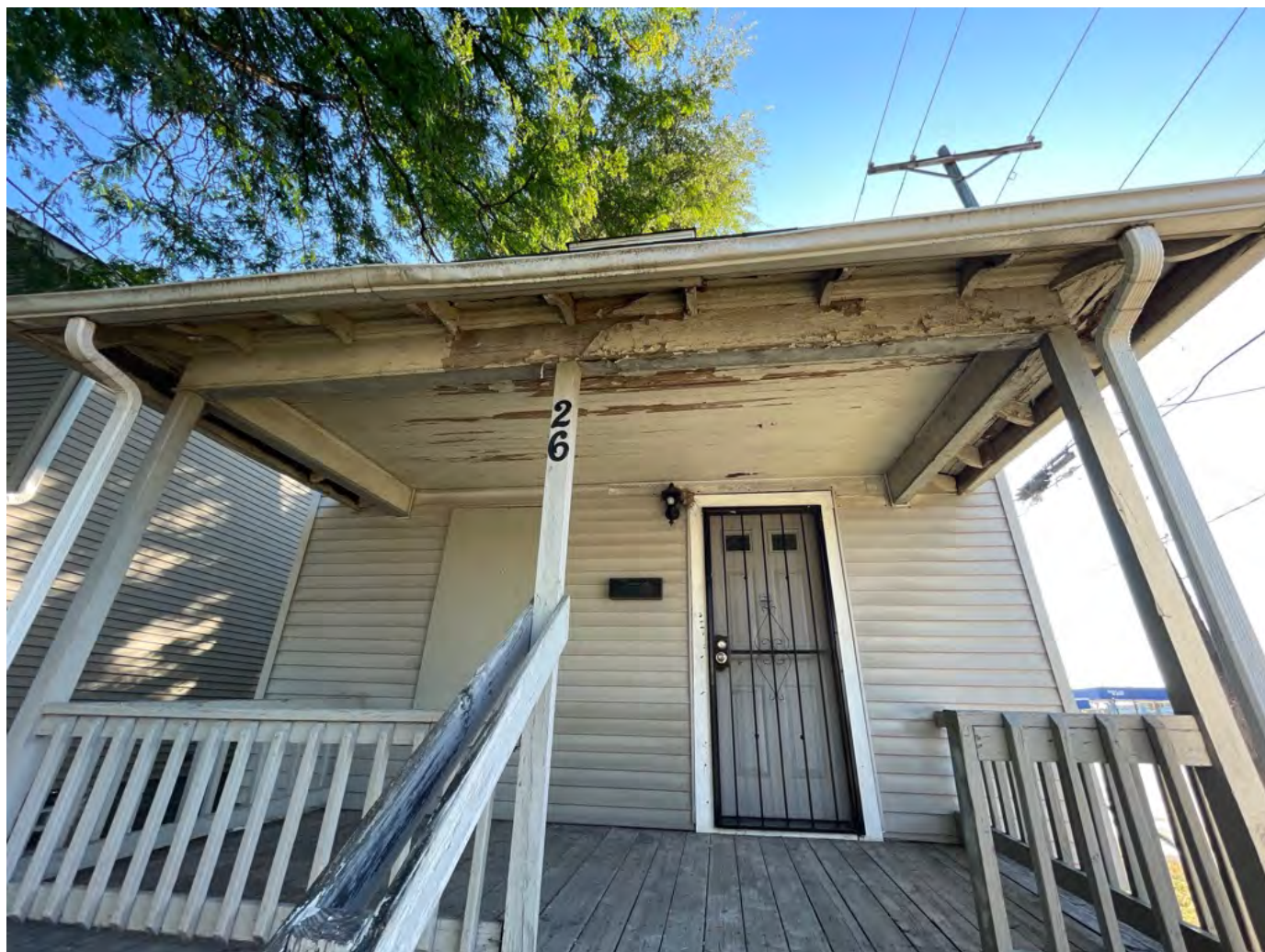
Vacant structure not boarded to code. Soffits detaching, damaged and/or otherwise in a state of disrepair. Bare, exposed wood surfaces.
