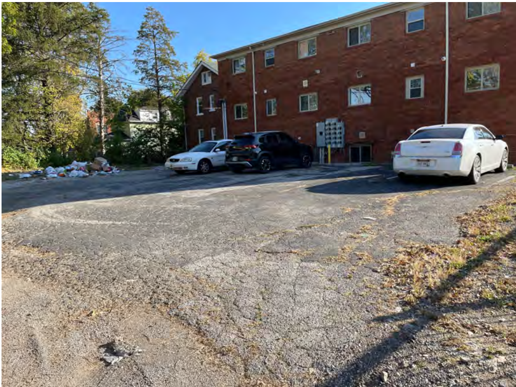
Parking/circulation area is cracked, damaged, and/or otherwise in a state of disrepairSolid waste
