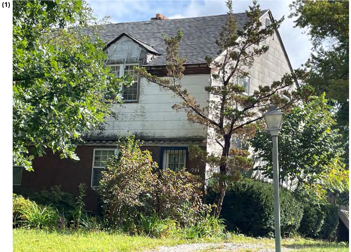
Sections of siding missing on front and south side of structure, as well as the sides of the dormers. Areas of exposed wood where siding is missing, on fascia boards, and around window trim. Rain carriers missing sections.
