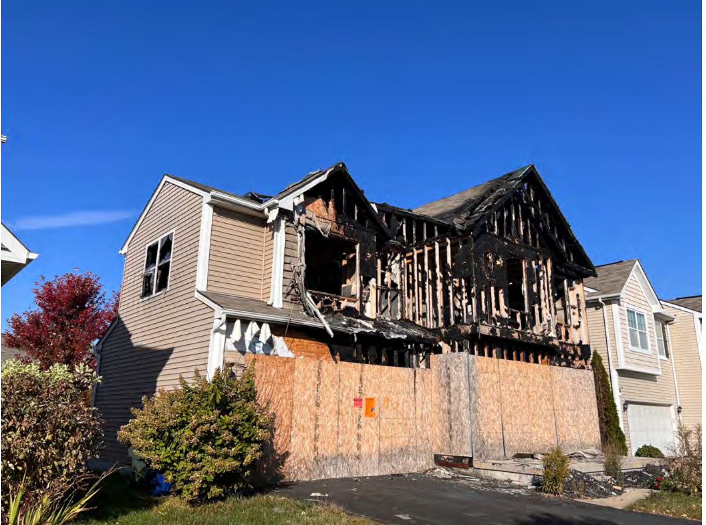
Vacant structure not boarded and secured to code. Severe fire damage throughout the structure including roofing, siding, soffit, fascia, trim boards, rain carriers, and broken windows. Boards covering the openings not painted. Address not clearly posted. Solid waste including debris created by the fire.
