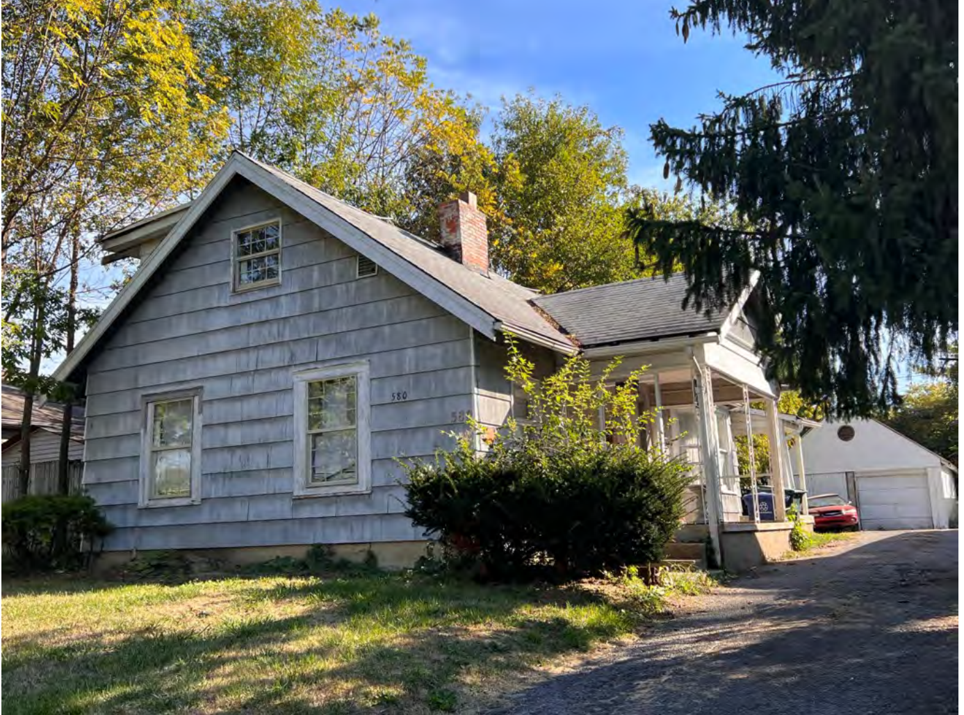
Exposed bare wood present on multiple areas of the main and accessory structures. Damaged asphalt in the driveway.
