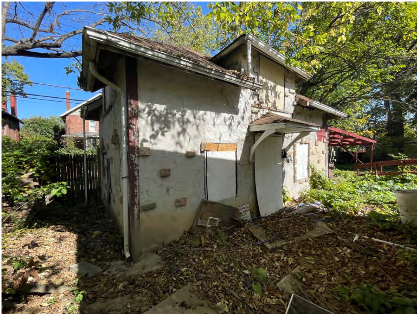
Bare, exposed wood throughout the accessory structure.
