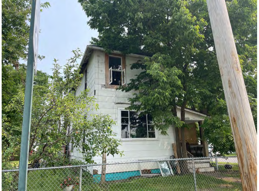
Bare, exposed wood surfaces present on exterior. Damaged and/or missing sections of siding. Improper exterior storage including window components.
