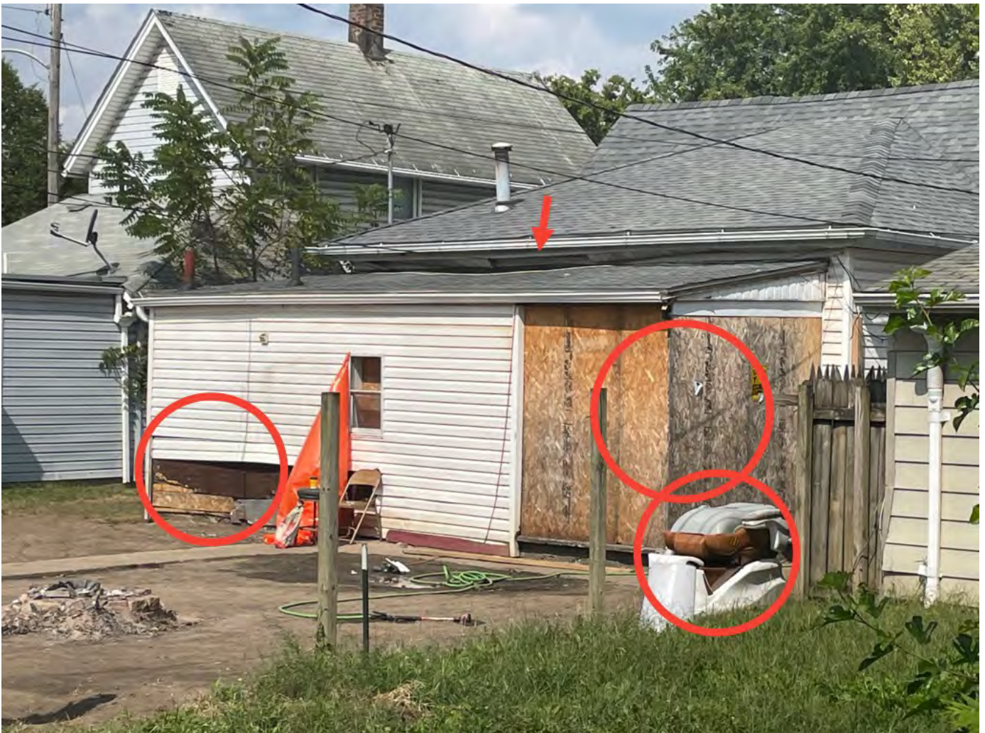
Damaged and missing siding. Missing soffit sections. Bare, exposed wood. Improper exterior storage.
