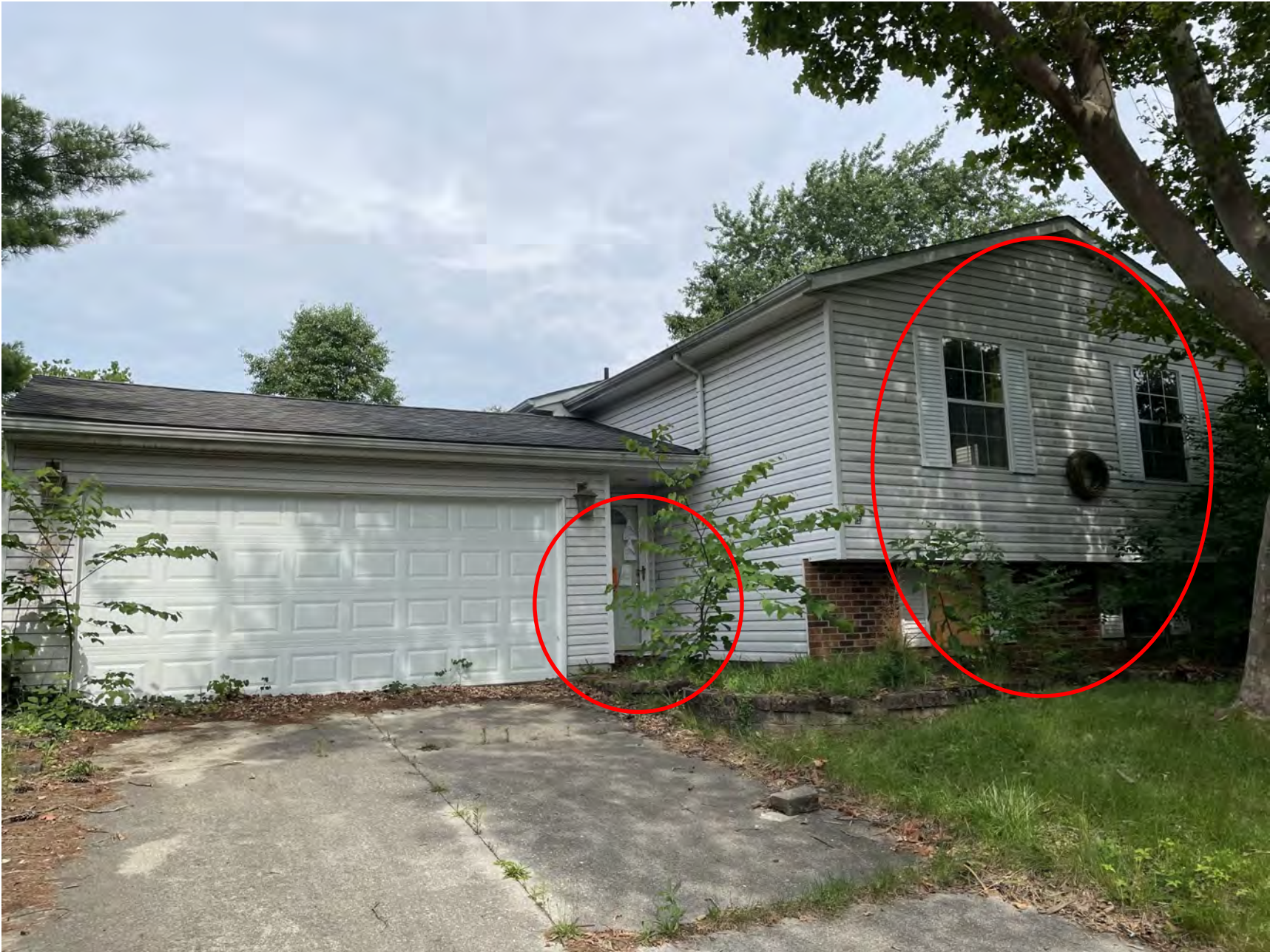
Vacant structure not secured to code.
