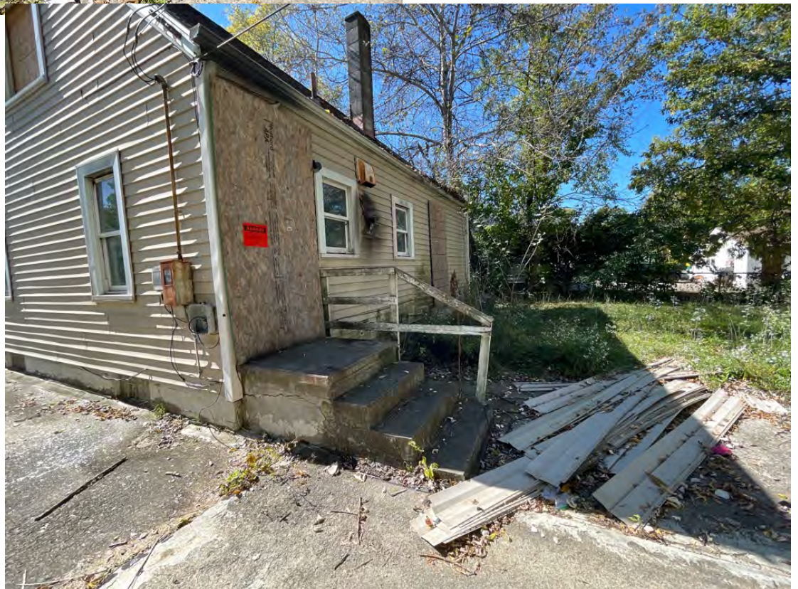
Vacant structure not boarded to code. Bare, exposed wood surfaces present on exterior. Damaged and/or missing sections of siding. Rain carriers full of debris. High grass/weeds. Solid waste.
