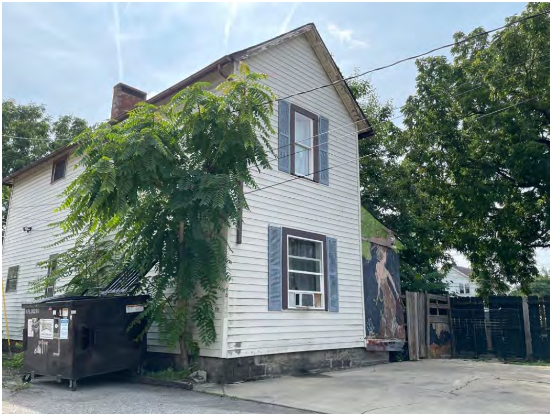
Address number for rear residential structure not clearly visible from the street or right-of-way. High grass and weeds. Solid waste.
