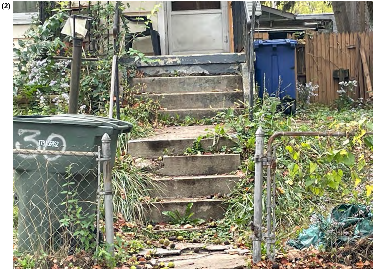
Front concrete service steps and walkway in disrepair and deteriorating.
