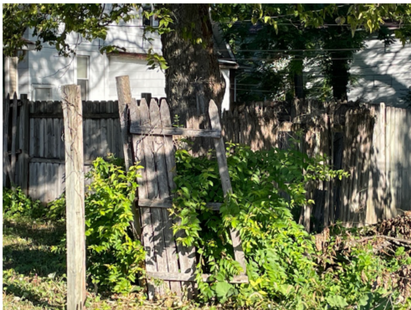
Fence in disrepair.
