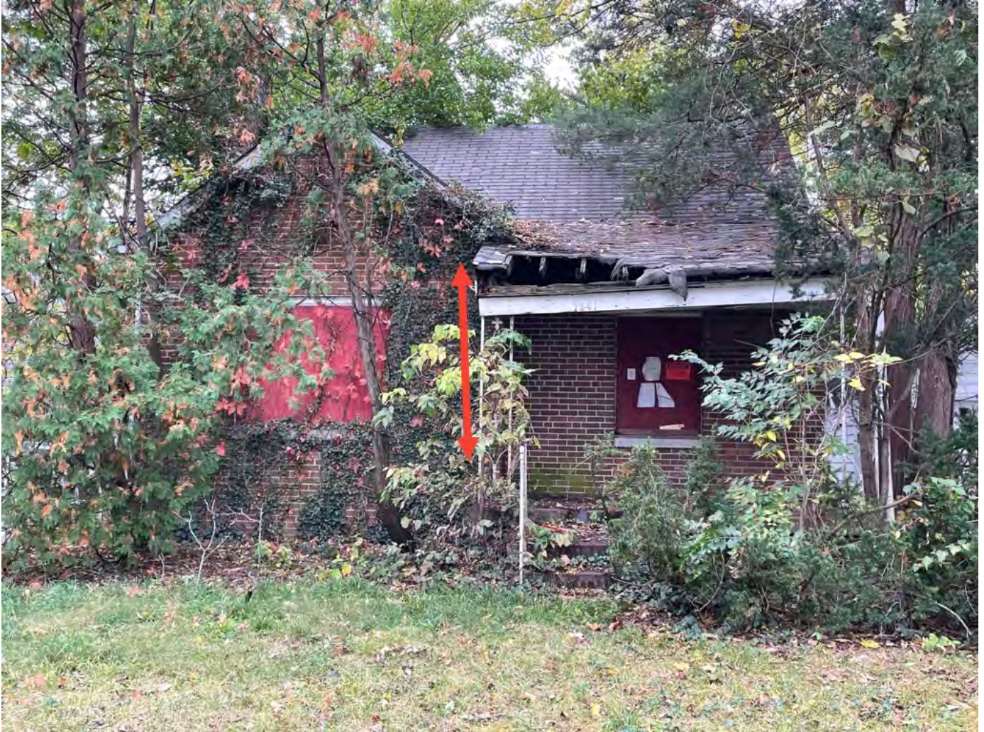
The porch roof has rotted, deteriorated bare exposed wood and has a large hole. There is bare wood exposed wood throughout. There is overgrown vegetation. Missing gutters.
