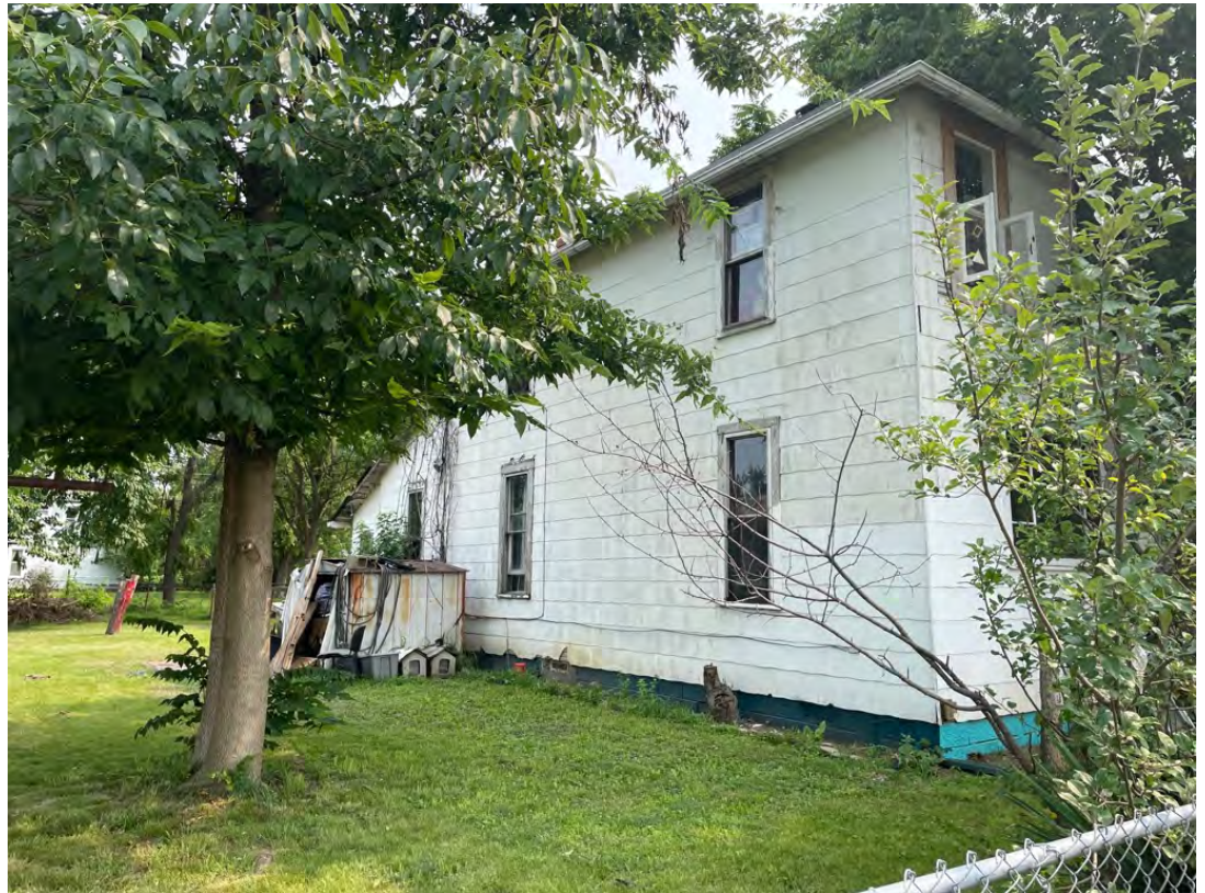
Bare, exposed wood surfaces present on exterior. Damaged and/or missing sections of siding. Improper exterior storage plastic containers, furniture and other miscellaneous items.
