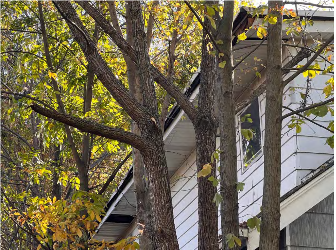
Missing and/or damaged sections of fascia and soffit on the north facing side of the main structure.
