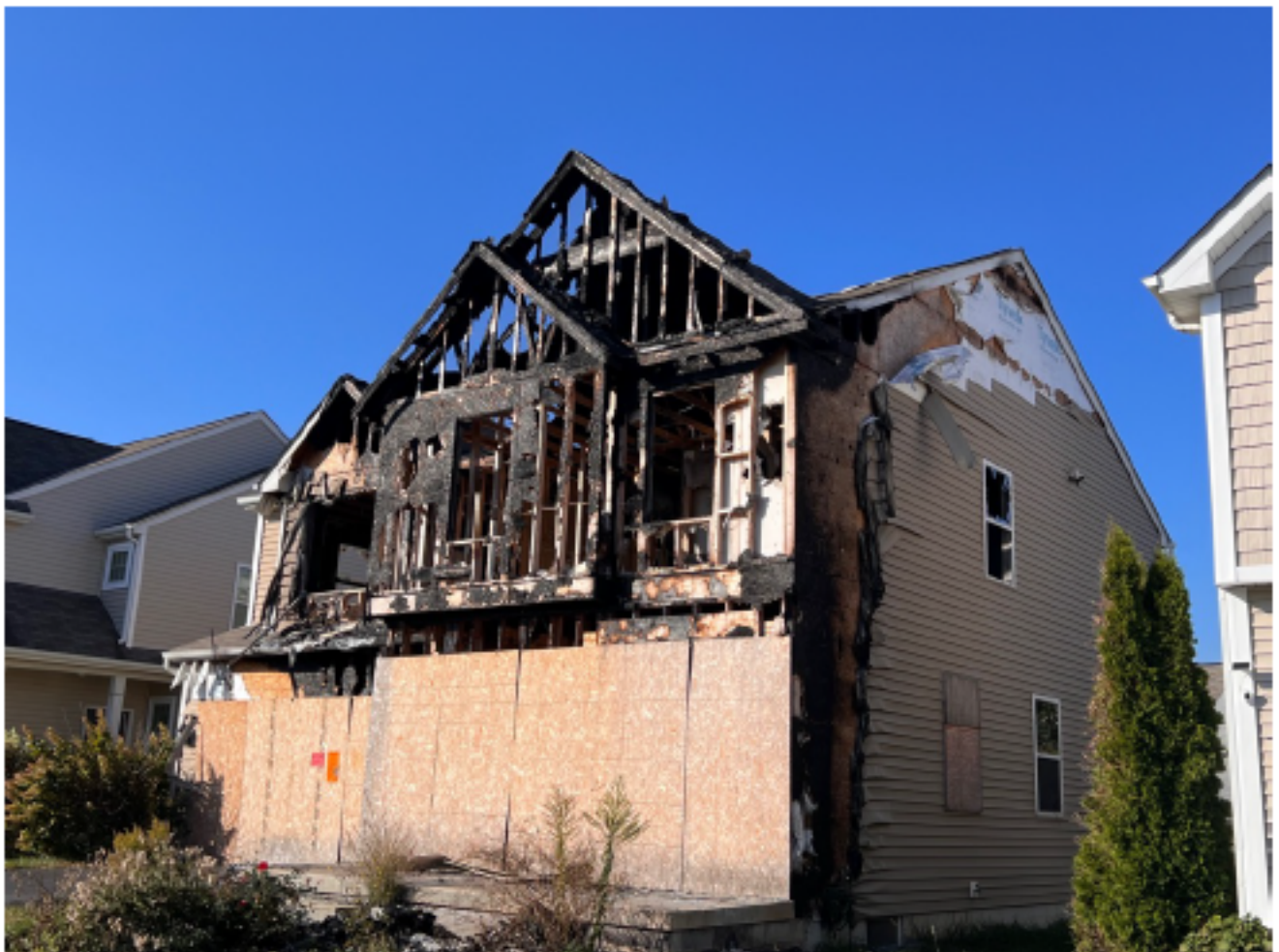
Vacant structure not boarded and secured to code. Severe fire damage throughout the structure including roofing, siding, soffit, fascia, trim boards, rain carriers, and broken windows. Boards covering the openings not painted. Address not clearly posted. Solid waste including debris created by the fire.
