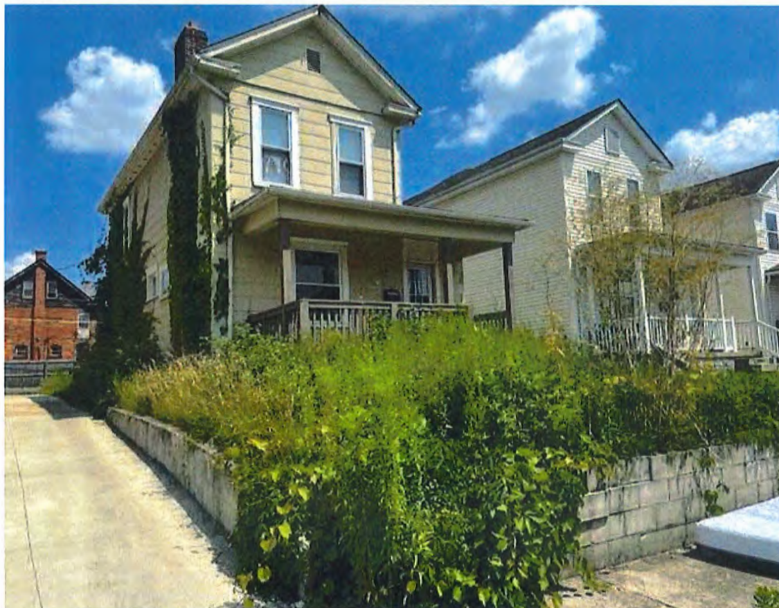
Violations observed: Not boarded to code, damaged retaining wall, trash and debris, high grass and weeds, rain carriers in disrepair
