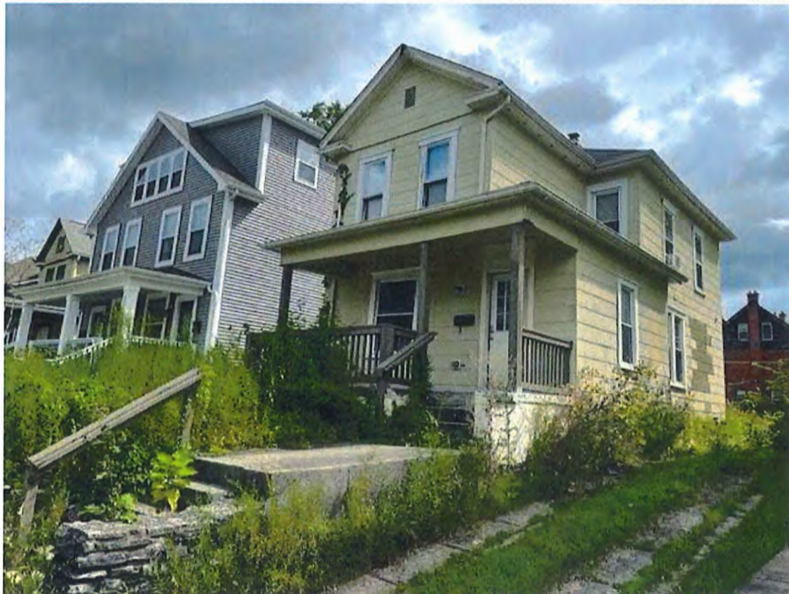
Violations observed: Violations observed: Not boarded to code, damaged retaining wall, trash and debris, high grass and weeds, rain carriers in disrepair
