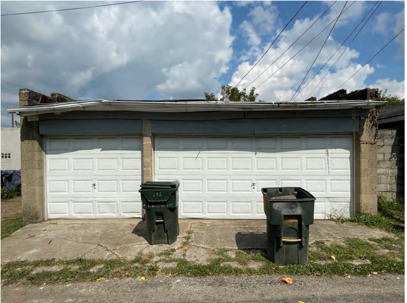
Damaged rain carrier. Missing downspouts.
