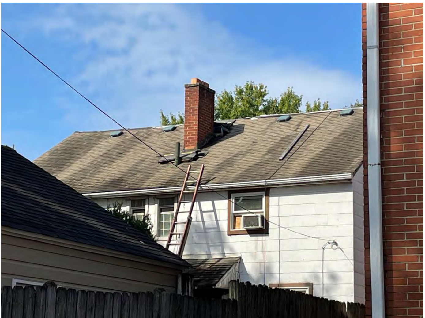
Roofing materials in disrepair. Loose materials stored on roof, and ladder stored on the exterior against the structure.
