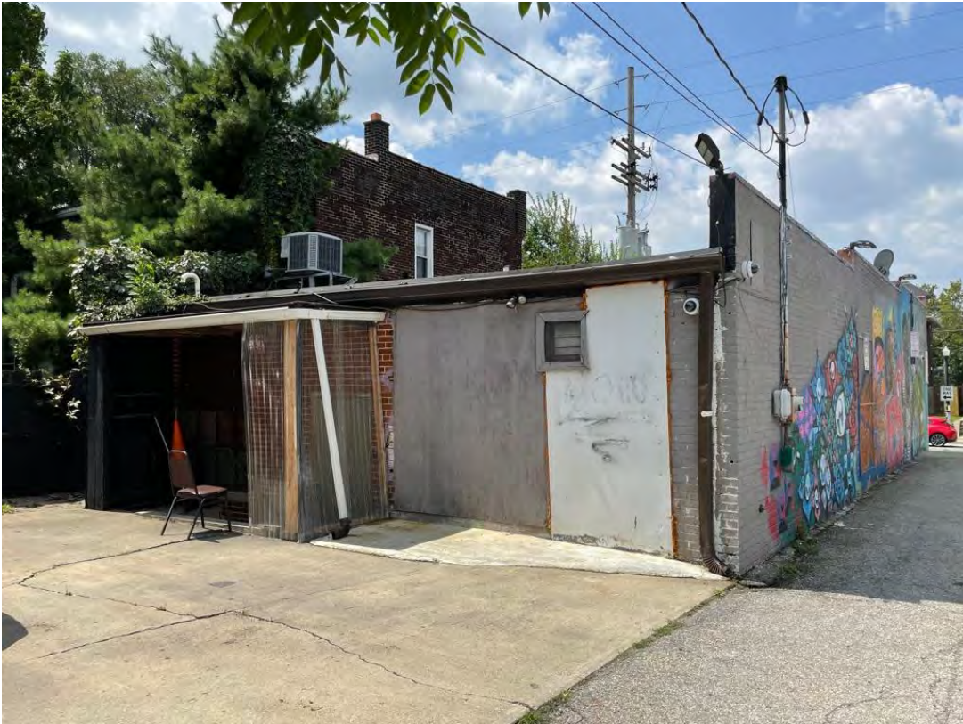
Brick corner contains mortar voids near the downspout.
