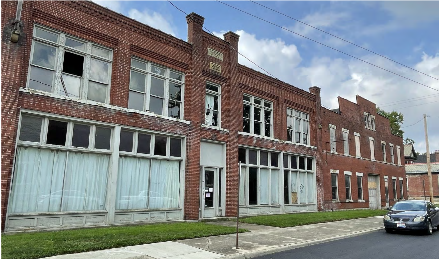
- Violations shown above: Not boarded to Code, bare and exposed wood, broken window, mortar voids throughout, graffiti.
