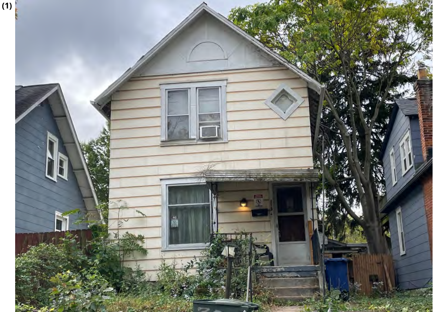
Soffit, fascia, and wood siding contain areas of exposed wood throughout. Front lamp post in disrepair. High grass and weeds.
