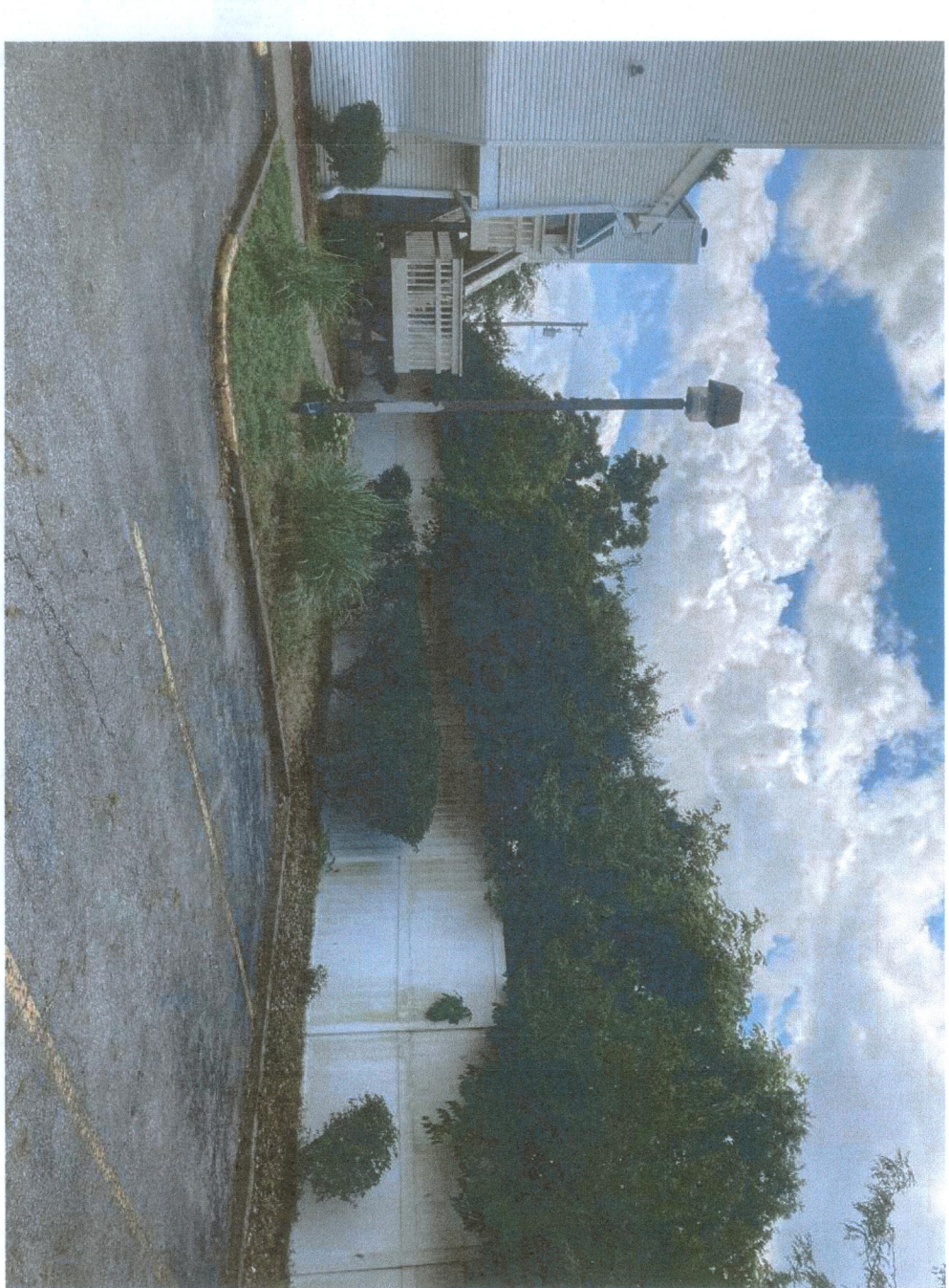
5 EXISTING LIGHT IN PARKING PENINSULA NOTE: TO BE WEEDED AND PRUNED AS NEEDED
